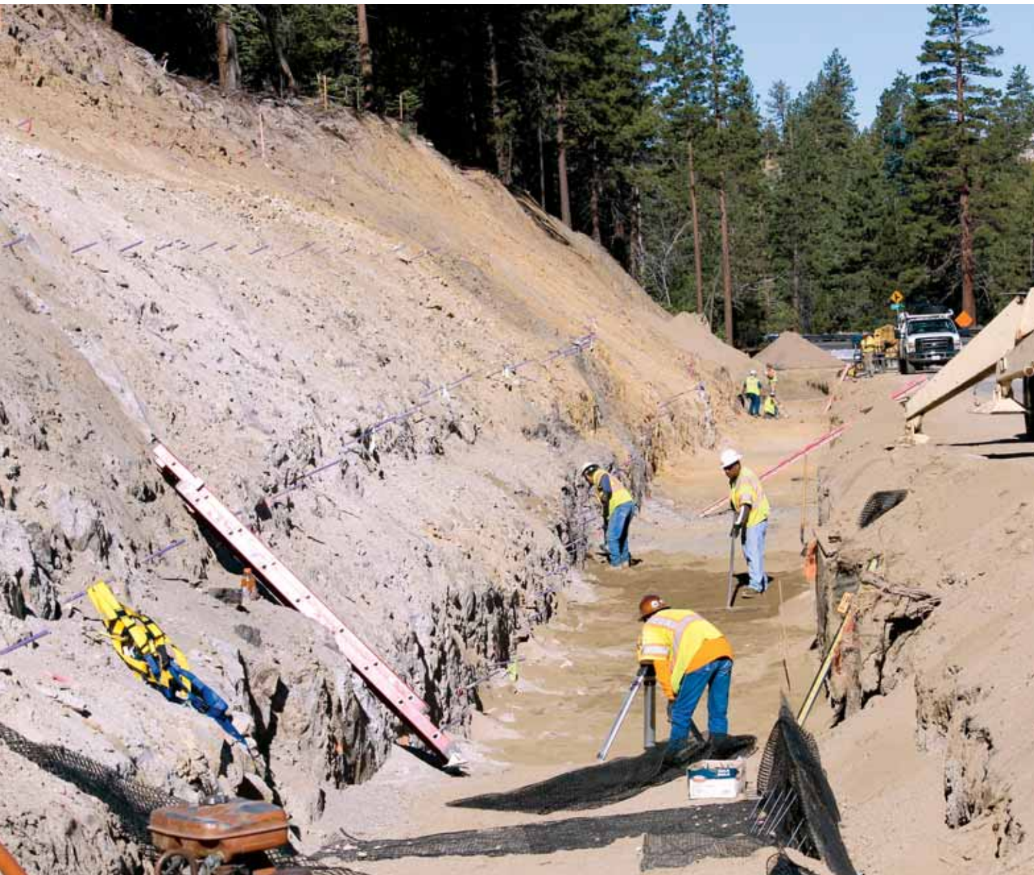
PHOTO 1 Rock anchor drilling commenced in the spring of 2012. Rock anchors were the linchpins of the project and their design was carefully considered to withstand the loads on the veneer soil slope.
