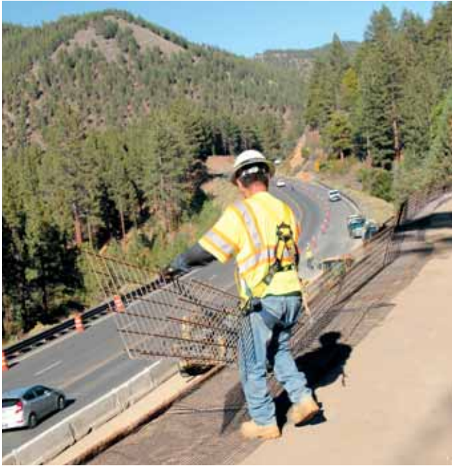
PHOTO 3 The welded wire forms were fabricated in conformance with ASTM A185 with w5.5 steel wire meeting ASTM A82 and measured about 10 feet long with a 22-inch front face (19-inch vertical rise) and an 18-inch base.
