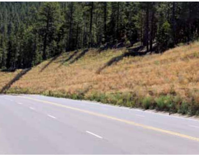
The slope along U.S. 50 near Lake Tahoe is now secure and stable. The project's life is expected to be in excess of 70 years.
