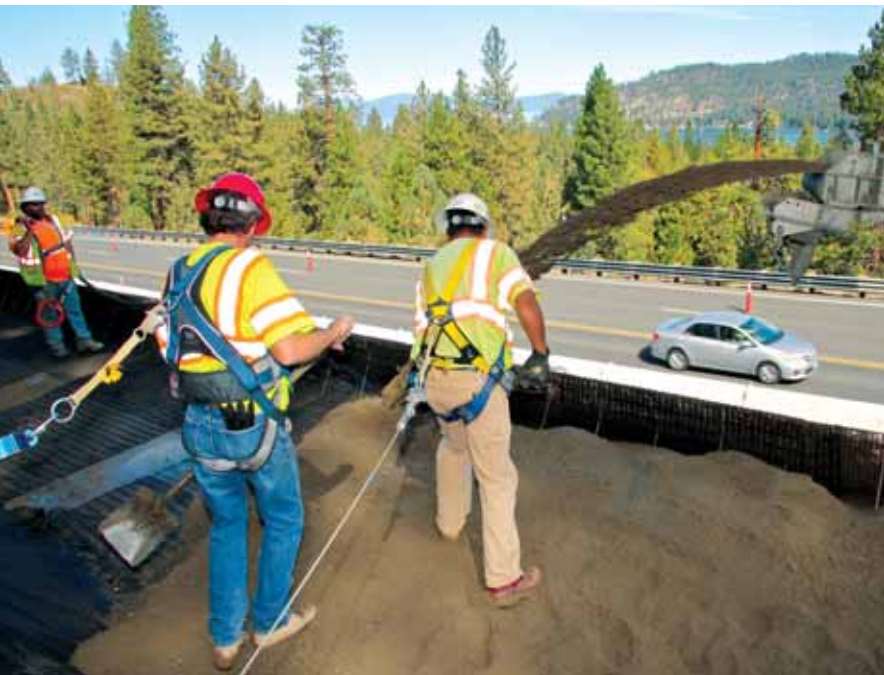
PHOTO 6 Backfill was placed using a portable conveyer to reach the higher elevations of the slope.
