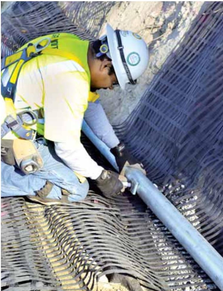
PHOTO 2 At each anchor location, a 6-foot-wide layer of geogrid was attached using a simple wrap connection around 3-inch diameter pipe.
