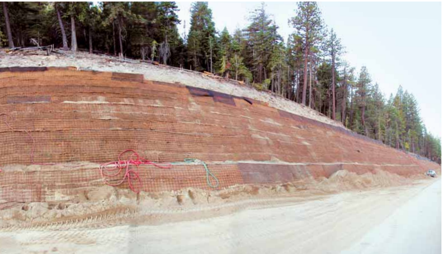
PHOTO 8 A wide-view lens captures the entire slope near project completion. This reinforced soil slope meets requirements for beauty and strength: Motorists are protected from rocks and soil in the road, and runoff has been stopped from crossing under the roadway and emptying into a nearby stream system that flows into Lake Tahoe.
